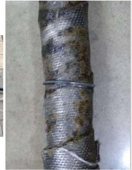
Tape is intact with blackening but keeping cable safe
