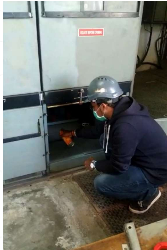
Panel Cable Entries
