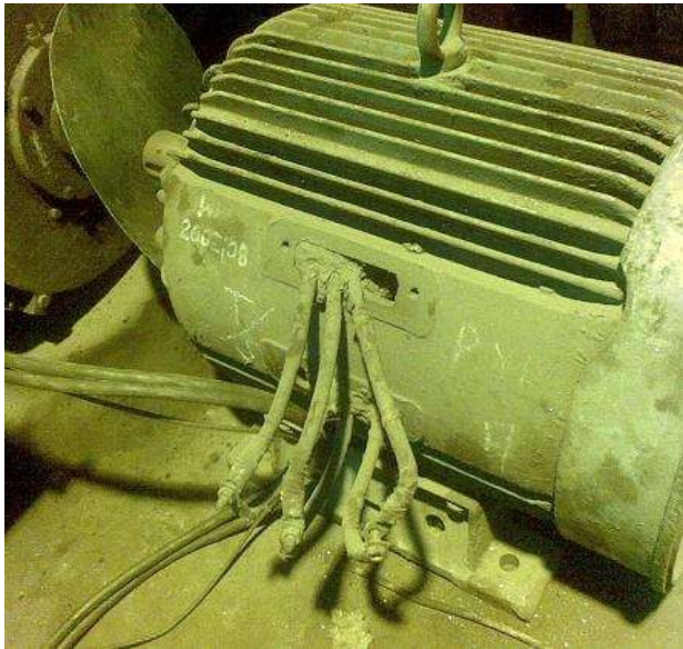
Improper Insulation leading to Dust and moisture
